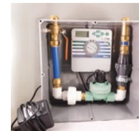
Irrigation Control Unit w/ fertilizer injector system
